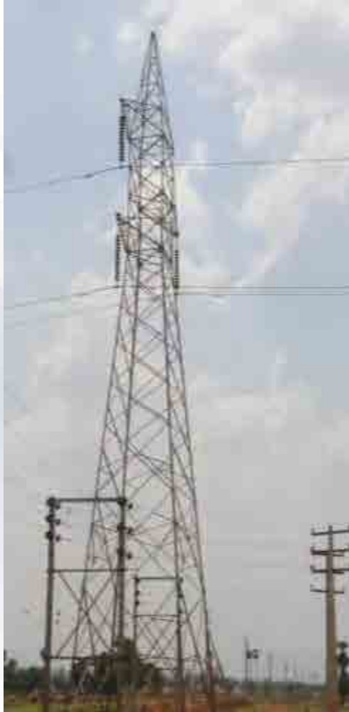
Power transmission lines
