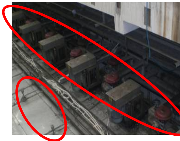
Fig-1: Dryer and control equipment
